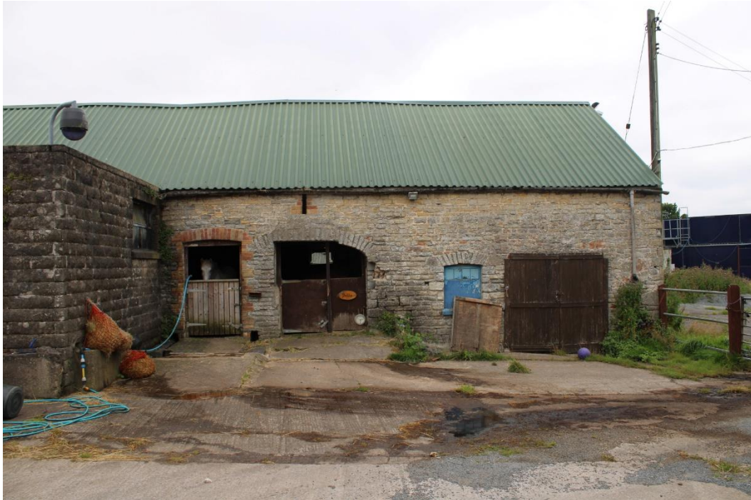
Photo 10: Looking west at northern end of western side of courtyard, showing present use as stables
