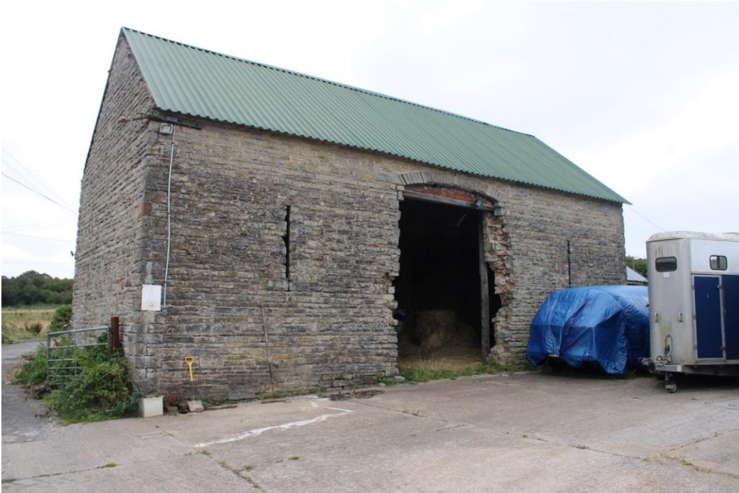
Photo 14: Looking southeast at western façade of threshing barn on eastern side of courtyard
