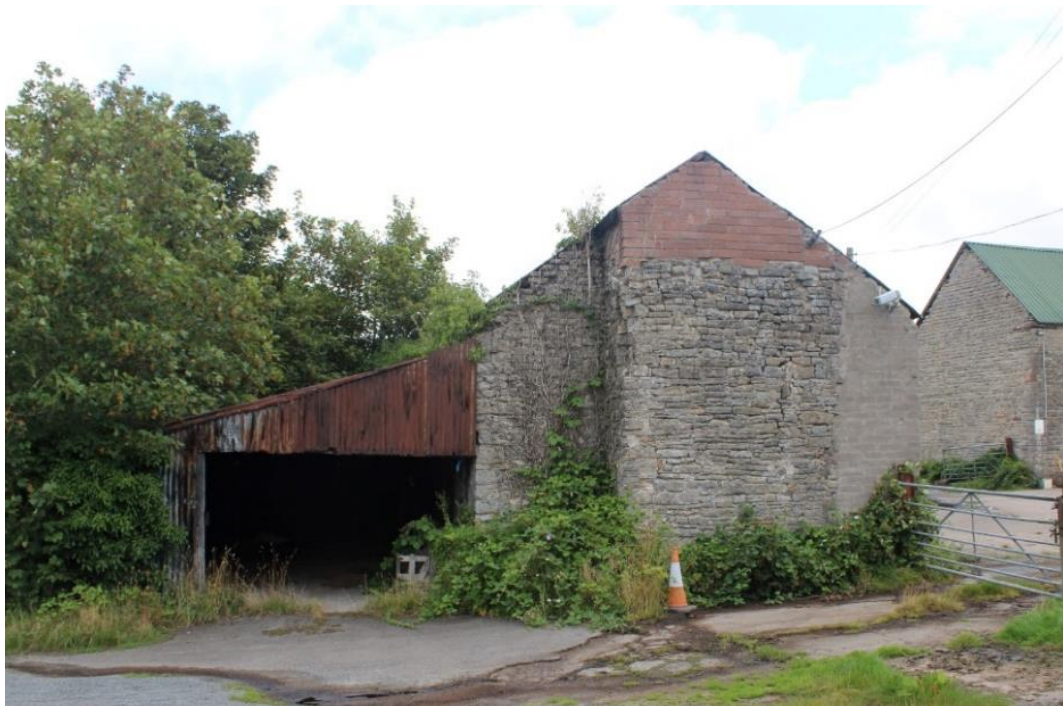
Photo 3: Western gable end of farmhouse with northern lean-to metal farmed extension, with chimney stack and rebuilt southwestern corner, and brick above
