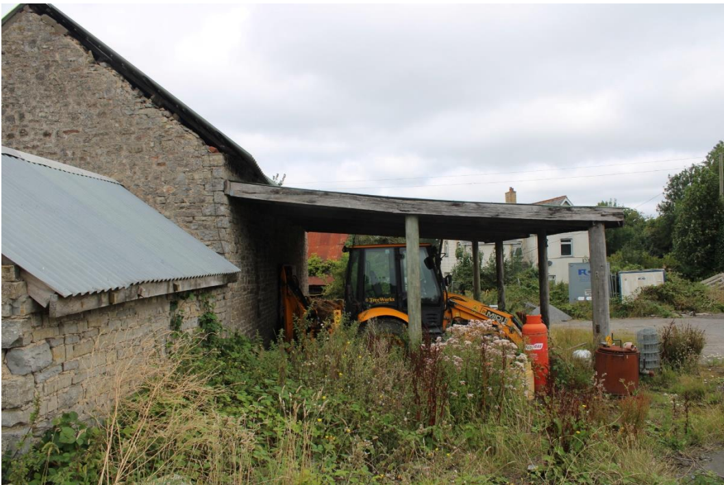
Photo 17: Looking south along eastern side of threshing barn and wooden lean-to extension on eastern side with modern farmhouse behind
