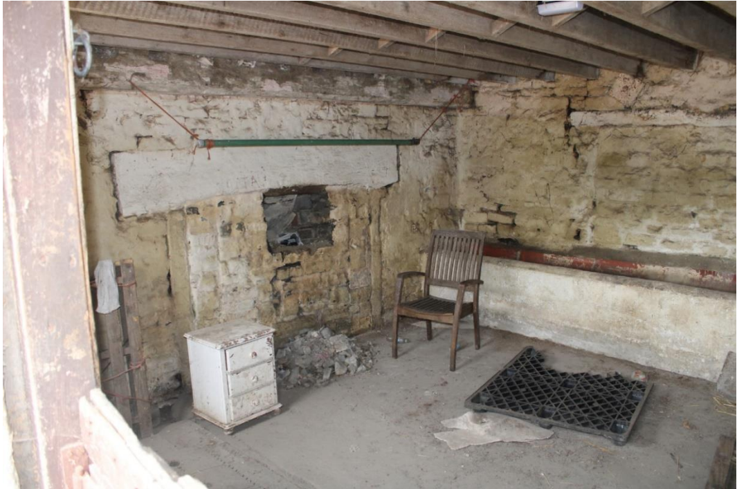
Photo 6: Looking northwest through western late 17 th extension of Lower Cosmeston Farm, showing infilled fireplace to left and infilled window to right.
