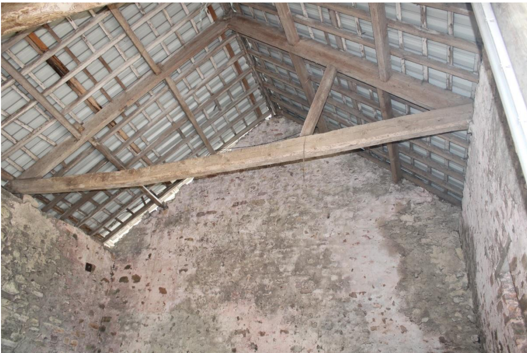
Photo 15: Looking south along interior of threshing barn showing roof structure and gable end
