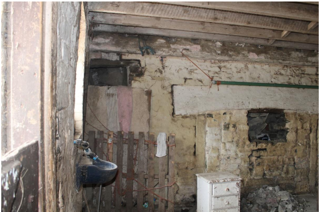
Photo 7: Looking west through the western extension of Lower Cosmeston Farm, showing original blocked doorway to first floor to left and infilled fireplace to right.
