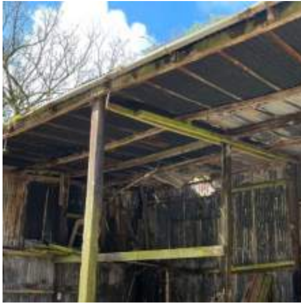
(4) Corrugated Barn in disrepair (to be removed)
