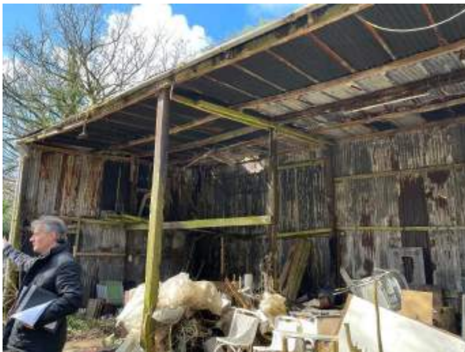
Large dilapidated corrugated barn to be removed and replaced with two smaller lodges
