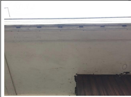
Photograph : Building 4 – Example of gaps under fascia boards between batons
