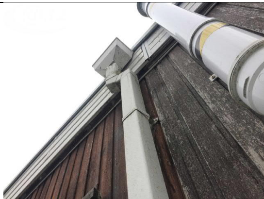
Photograph : Building 1 – gap behind fascia board
