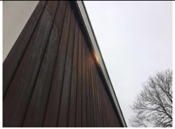
Photograph : Building 1 – north face. Example of gaps under fascia boards between batons
