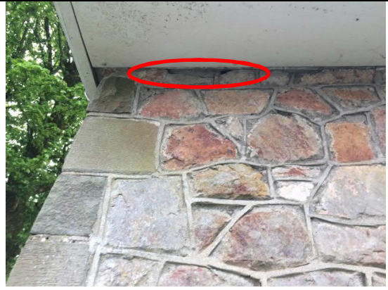
Photograph : Building 2 – gap between stonework and fascia board
