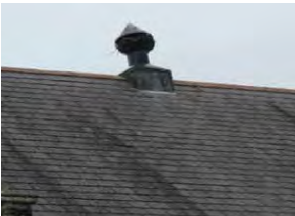
Roof vent with evident nesting bird material
