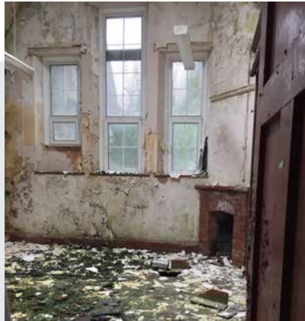
Fig 9 (Above): Existing interior of the school buildings, showing significant signs of dilapidation
