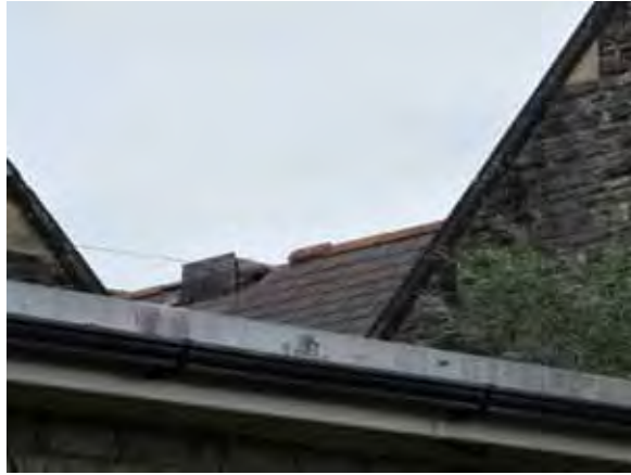
Missing ridge tiles providing potential roost feature
