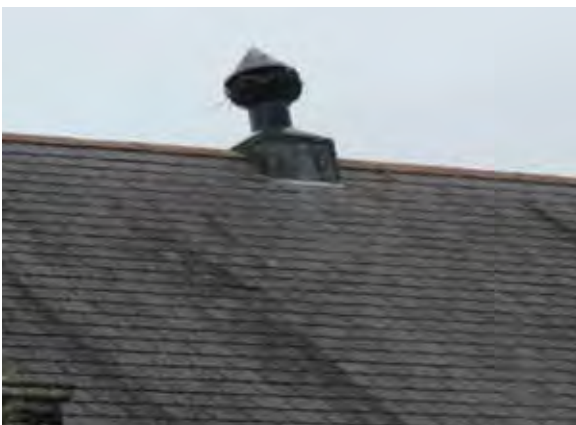
Roof vent with evident nesting bird material
