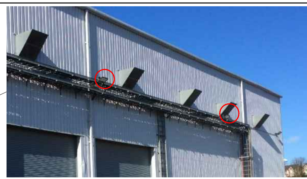
Image 1.1 showing floodlights mounted at 7.5m along exterior cladding of Wood Processing Warehouse
