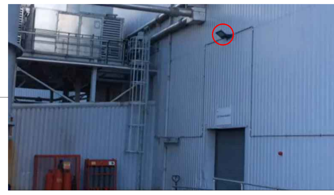
Image 1.3 showing floodlight (annotated) above vehicle entrance to Main Processing Building
