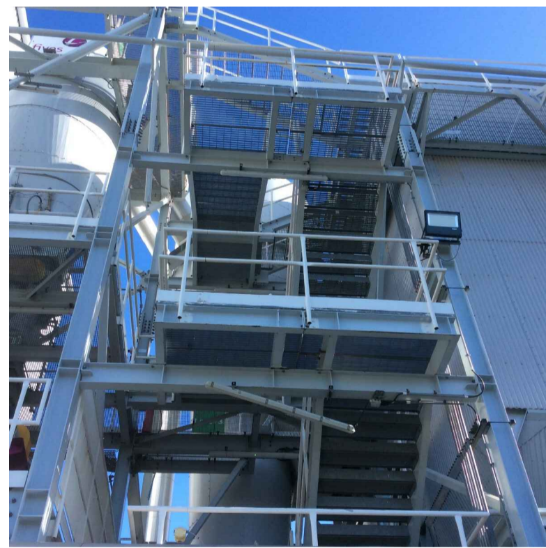
Image 4.3 showing floodlight mounted on third floor of bag house
