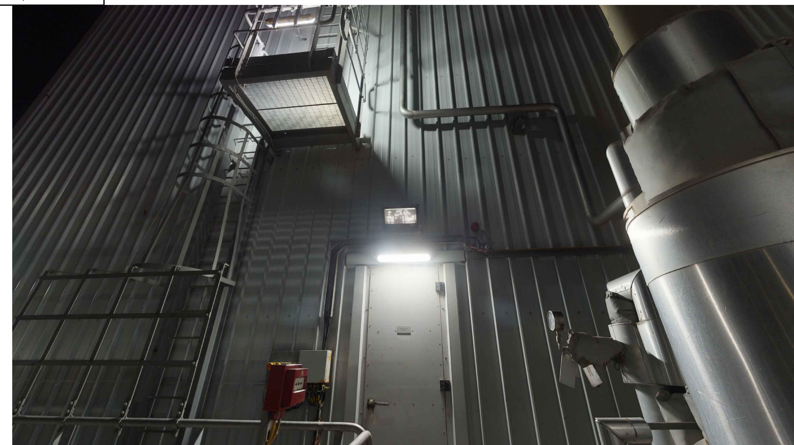
Image 5.1 showing floodlight mounted over batten luminaire above first floor doorway into fan units
