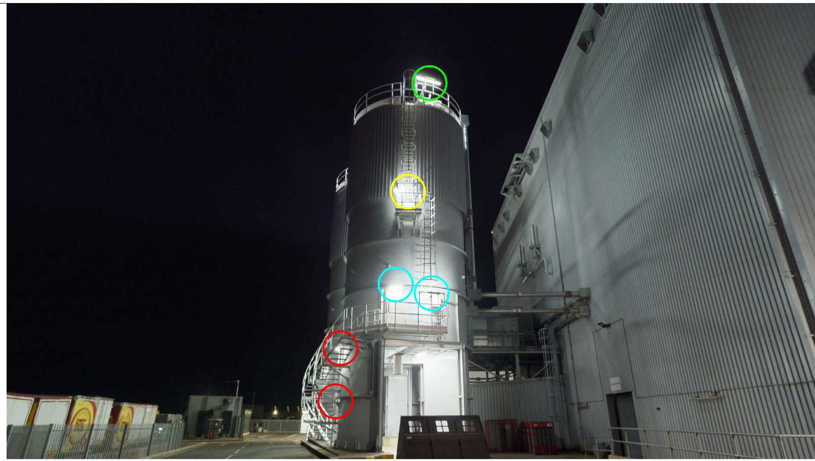
Image 3.1 showing batten type luminaires on northern ash silo annotated with circles. First ladder level luminaires in blue, mid ladder level luminaire in yellow, top of silo in green
