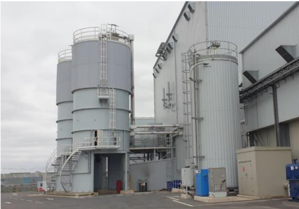
Figure 5.3: Enclosed Ash Silos showing sealed fill pipes and enclosed discharge
