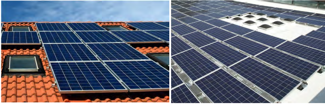
Figure 7 example SPV array installations
