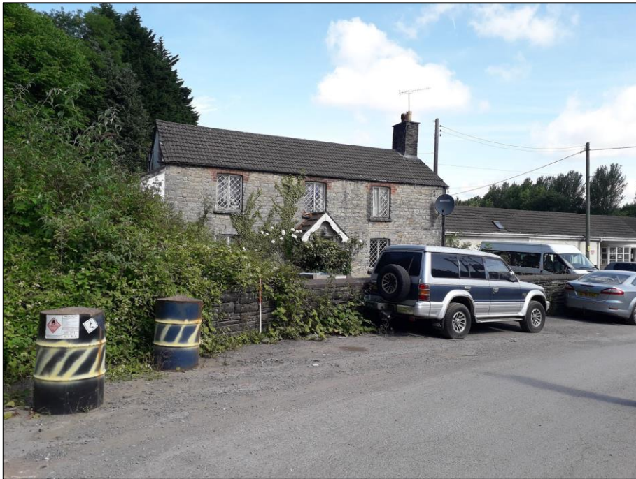
Plate 9. View to south of north facing elevation of Leckwith Bridge House (LQ001) (Scale: 0.5m divisions)
