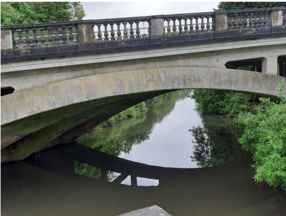
Photograph B - Leckwith Road bridge which is elevated above the site, over the River Ely which bounds the site to the east (WSP, June 2019)
