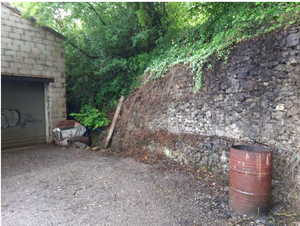
Photograph H - Gabion wall along the western boundary in the centre of the site (WSP, June 2019)
