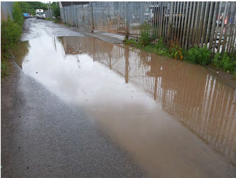
Photograph F - Large areas of ponding across the site following rainfall (WSP, June 2019)
