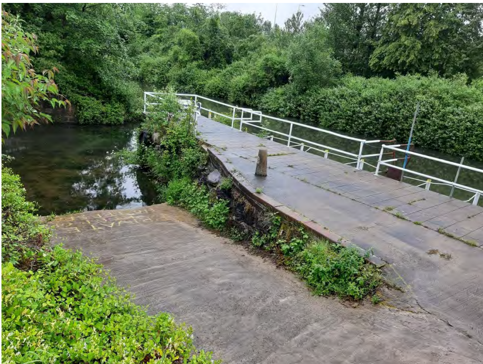
Photograph P - Slip way on the River Ely in the site east of the site (WSP, June 2019)
