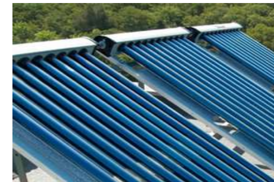
Figure 3: Solar thermal hot water panels.
