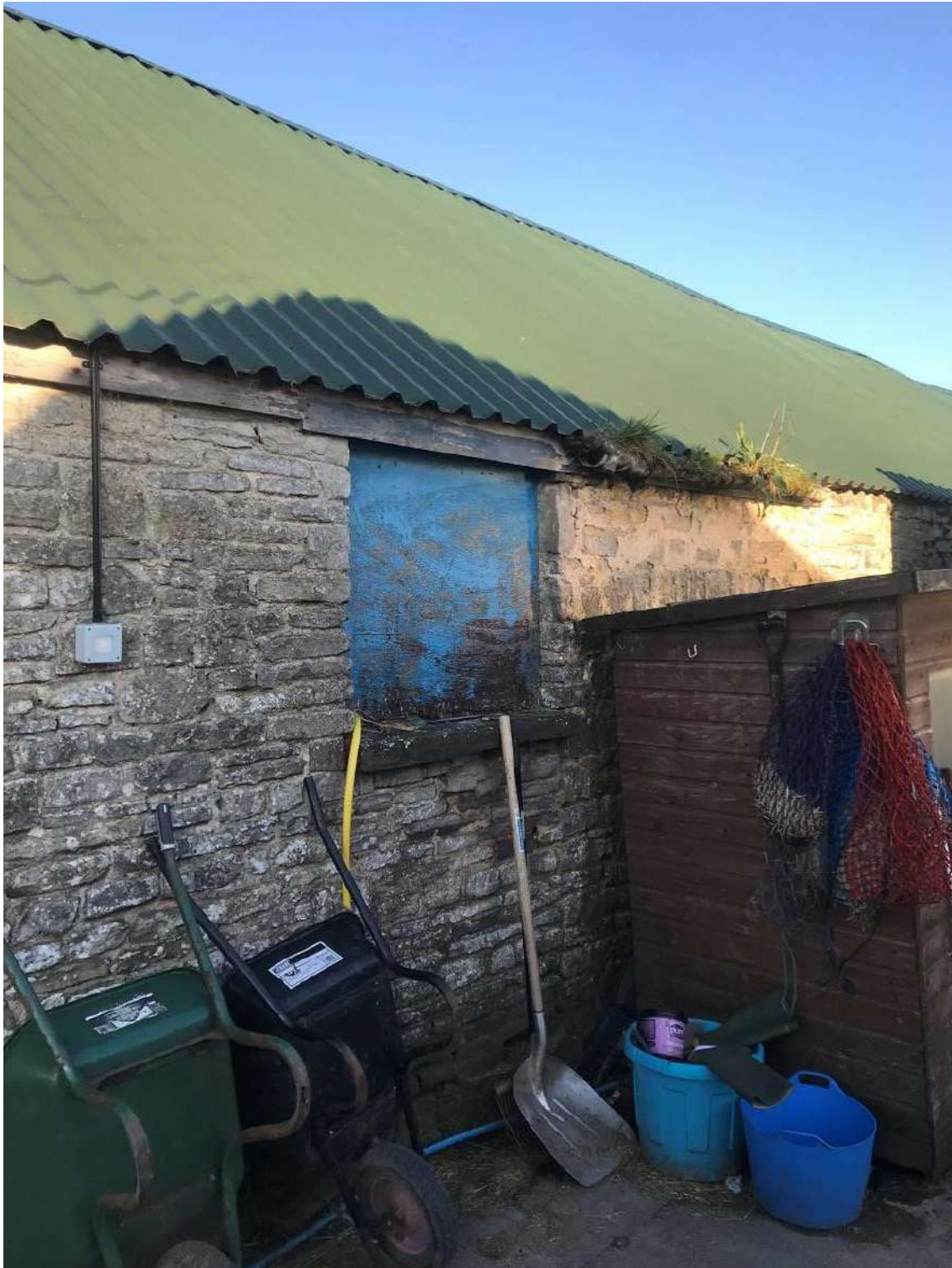
Image EDP 21: Close-up of the northern extension to Structure C, here highlighting that this element of the building has two principal elevations.
