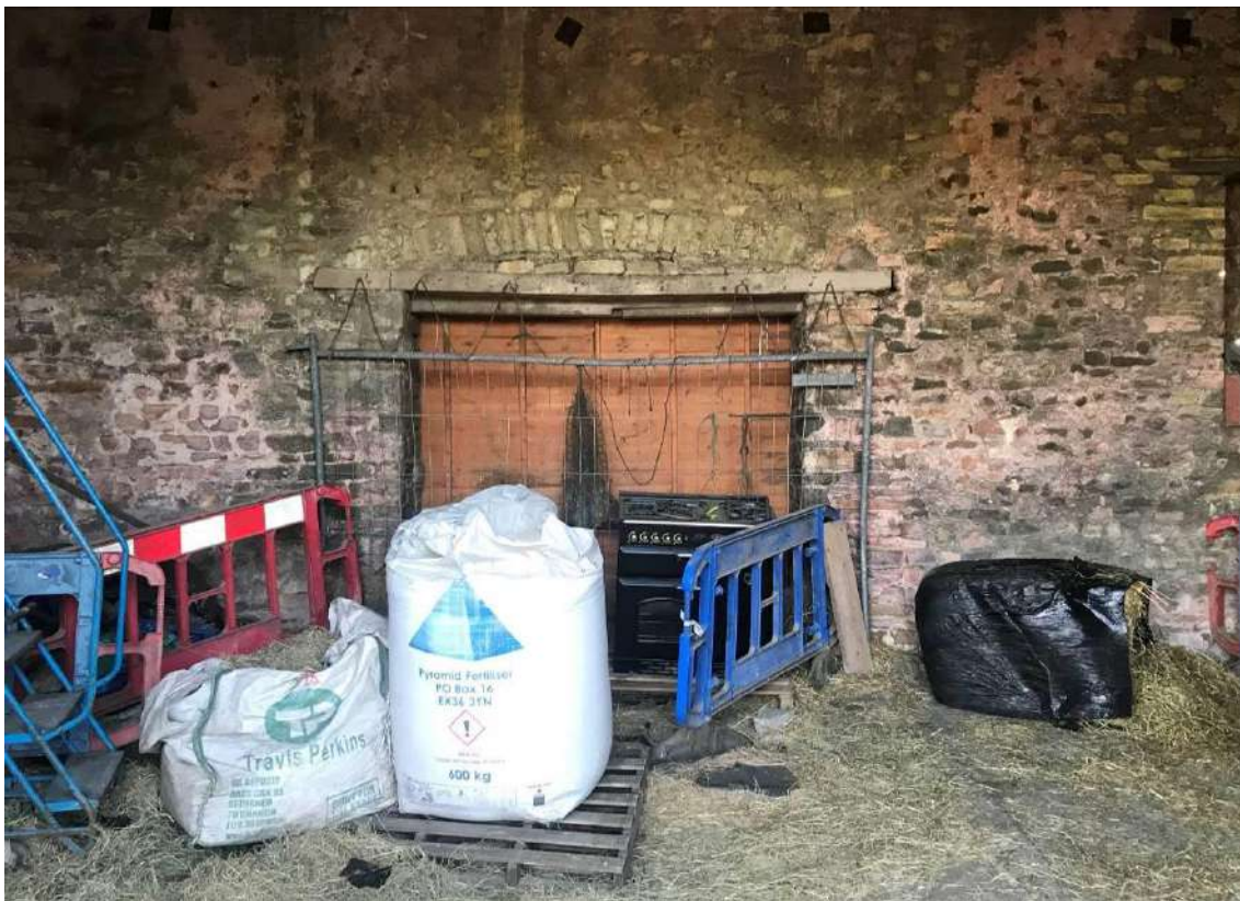
Image EDP 16: Close-up of the eastern cart opening from within the building, showing the form of the relieving arch in particular.
