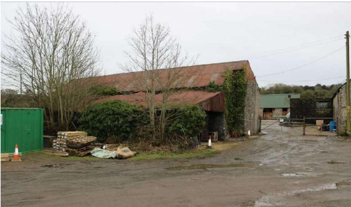
Image EDP 2: View of Structure A looking south-east from the old course of Lavernock Road and showing the projecting chimney stack at the western end.
