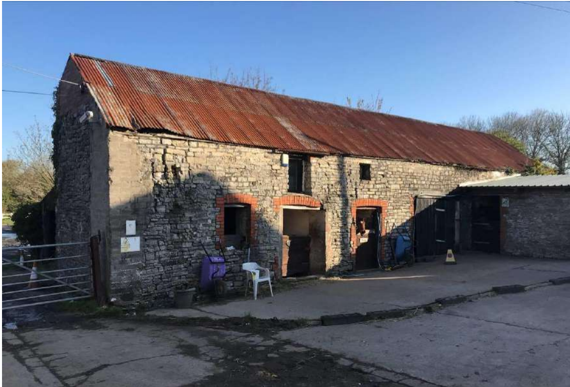
Image EDP 3: View of Structure A looking north-east from within the farmyard and illustrating the extent of adaptation associated with the house's conversion to a stable block.
