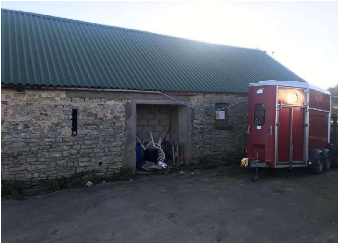
Image EDP 19: View of the east-facing elevation of Structure C, here highlighting the extent and character of the later northern extension.
