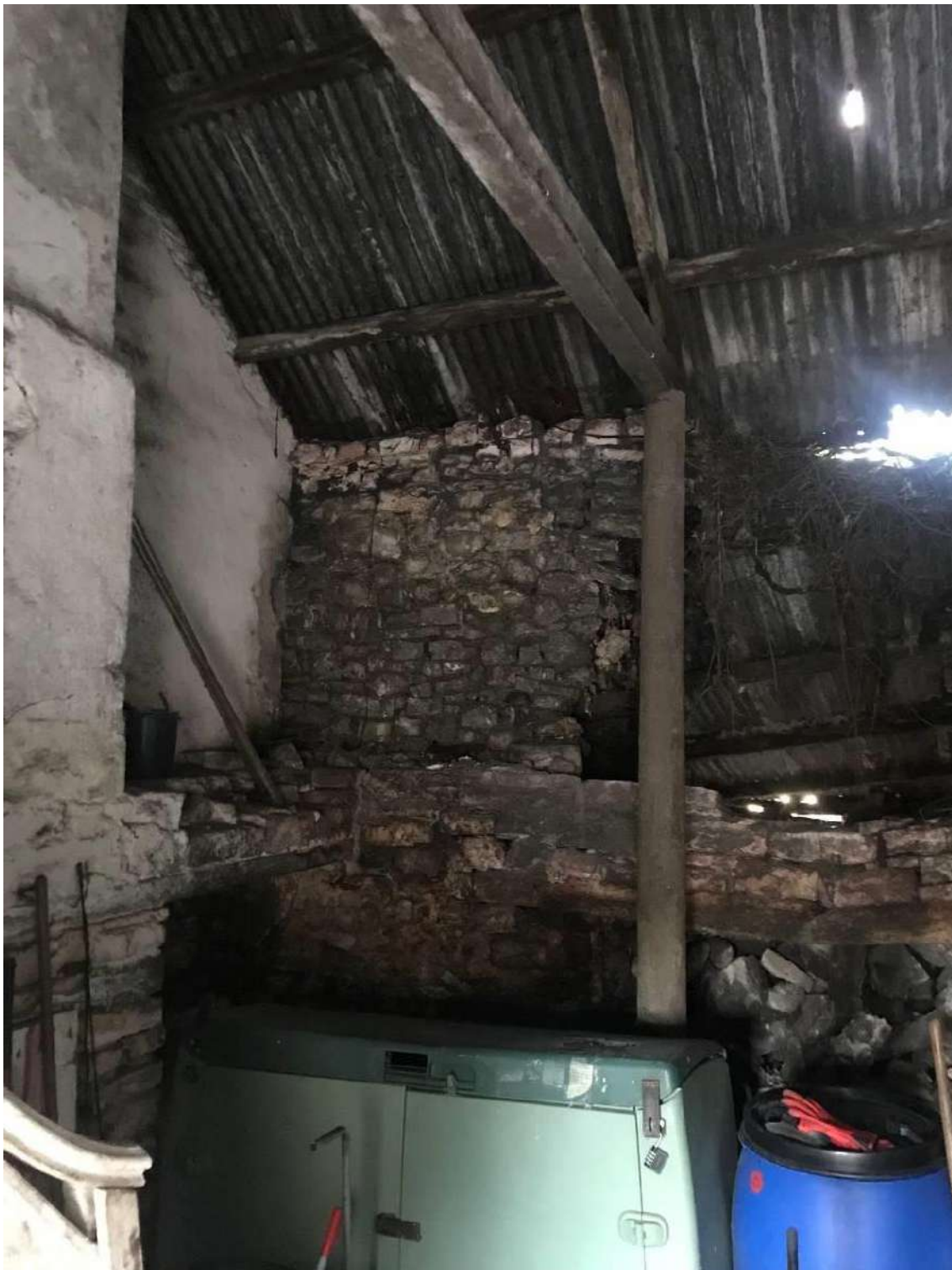
Image EDP 8: View of the internal space within the earliest element of Structure A, here looking north-west to the door opening on the opposite side of the chimney stack.
