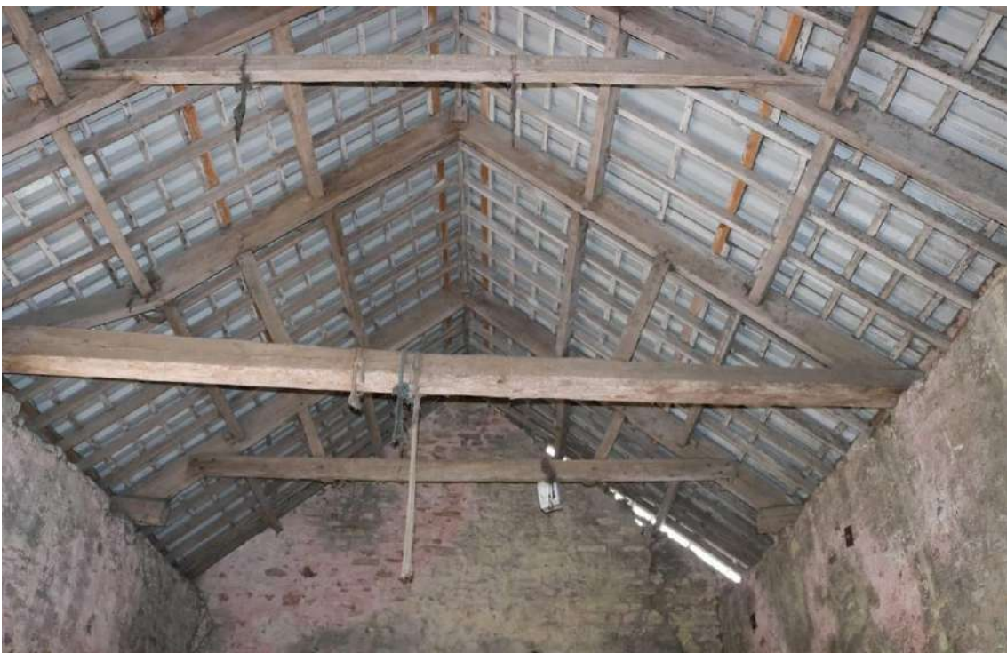
Image EDP 18: View of the interior of Structure B, here looking north towards Lavernock Road and highlighting the currently variable condition of the original roof structure.
