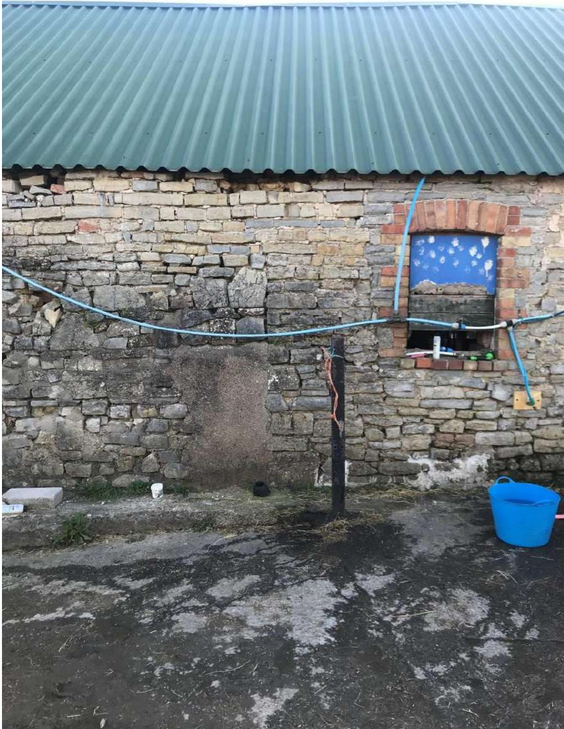
Image EDP 20: View of the east-facing elevation of Structure C, here highlighting the extent and character of the later southern extension.
