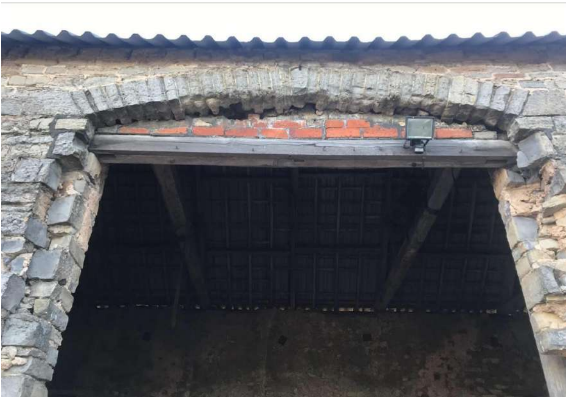
Image EDP 17: Close-up of the eastern cart opening to Structure B, looking east from within the farmyard and showing the impact of secondary alteration.
