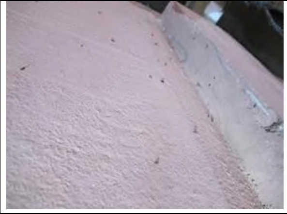
Bat droppings on wall interior – building 8
