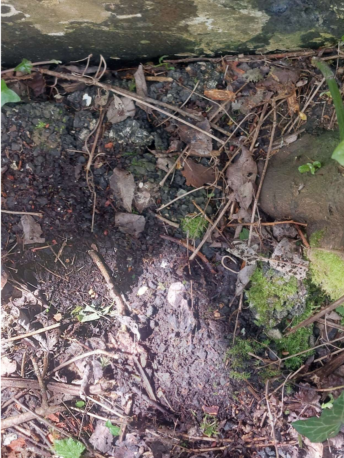
Photograph 7. Direct physical damage caused to hard surfacing by T44
