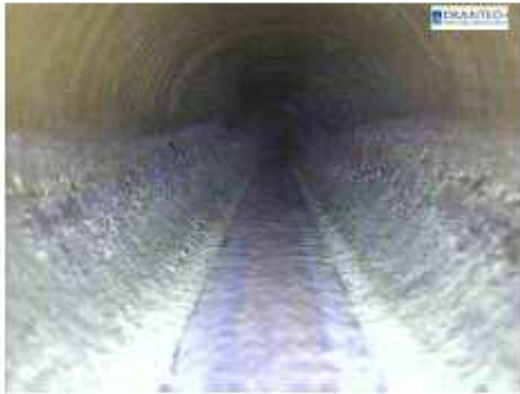
1, 00:02:52, 2.02 m Survey abandoned, Line needs cleaning - Spinning on grease
