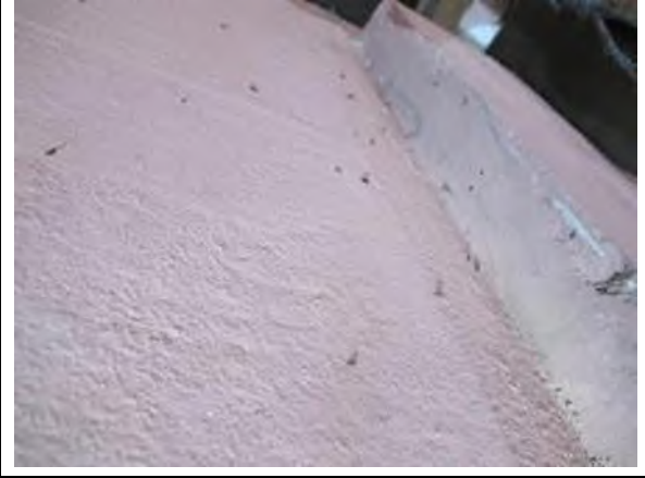
Bat droppings on wall interior – building 8
