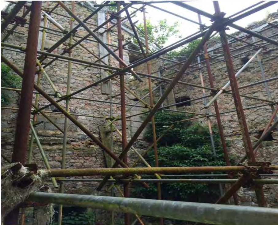
(Figure 13. View of the interior of Great Frampton farmhouse showing its deteriorated and fragile condition)
