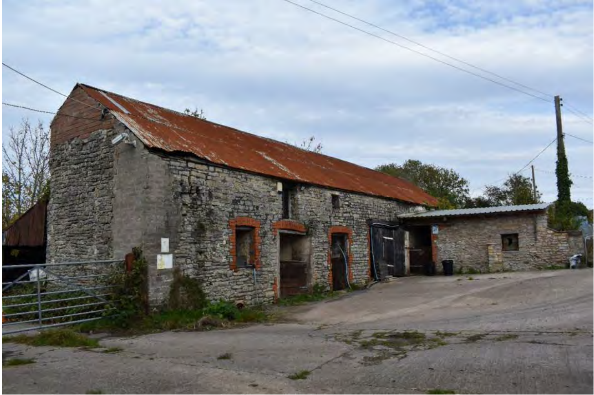
(Figure 2. View of Lower Cosmeston farmhouse from its south-west angle showing some of its later alterations and the Victorian period east-annex)
