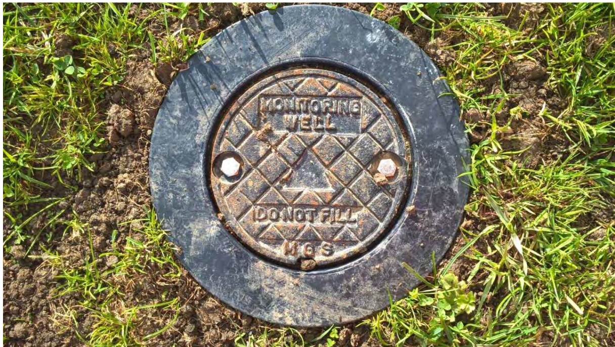
(Gas and groundwater monitoring flush cover)
