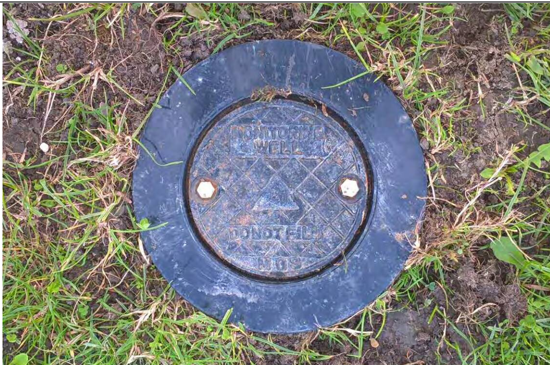
(Gas and groundwater monitoring flush cover)
