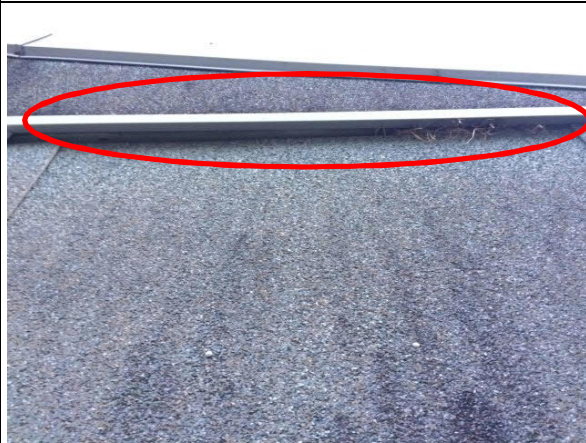
Photograph 3: Building 2 – South face. Roost entry / emergence location, beneath gable end fascia board. This feature is also used by nesting house sparrow (nest material can be seen).
