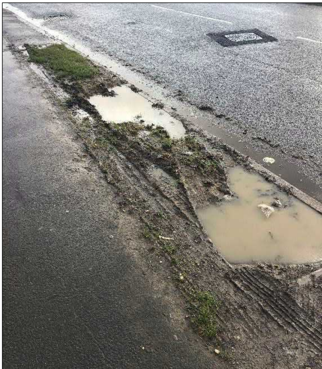
Figure 2-5: Damage to Highway Verge caused by Vehicle Parking
