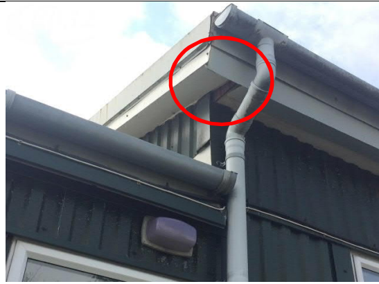
Photograph 23: Building 1, gap under fascia boards.
