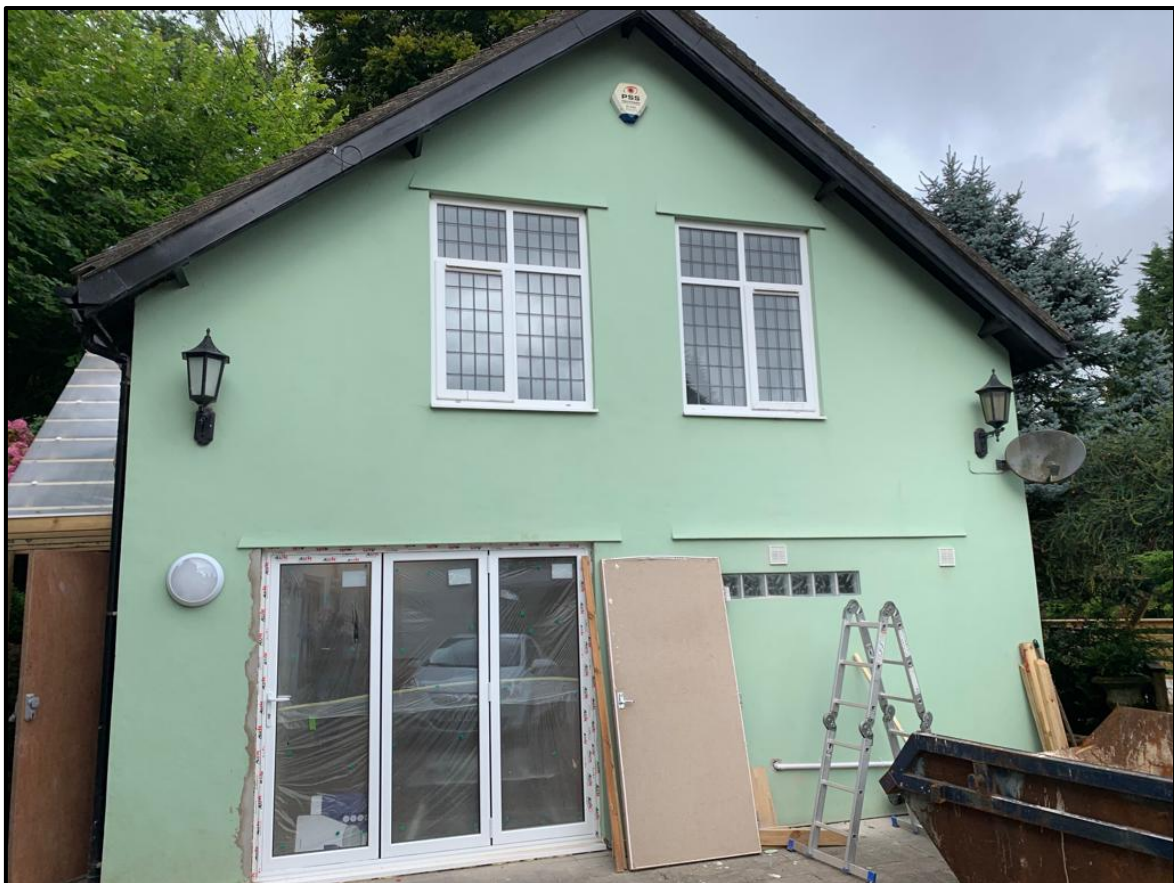
Figure 1. The Annexe, undergoing minor alterations in readiness for the start of the school term.
