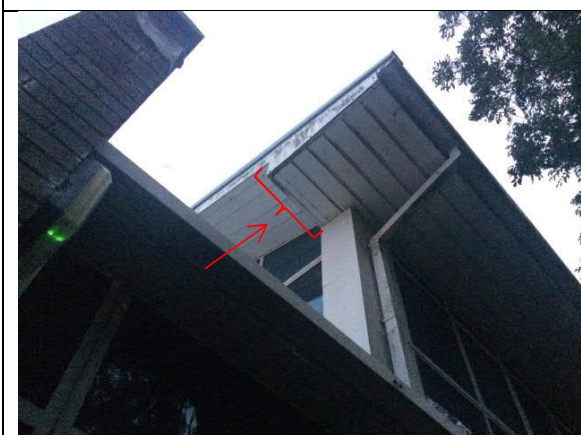
Photograph 5: Building 6 – north-east corner. Possible roost exit/re-entry point on edge of soffit. But this edge cannot be seen from ground.
