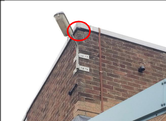
Photograph 44: Building 10, a close up of the bat feature identified in Photograph 43.
