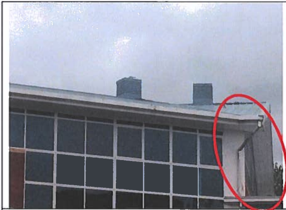
Photograph 7: Building 6 – Soffit box on west end. Possible roost exit/re-entry point along this edge, or where lower roof of B5 joins B6.
