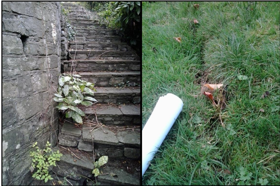
Plate 2.3. Evidence of Ground Movement during October 2015 visit.
