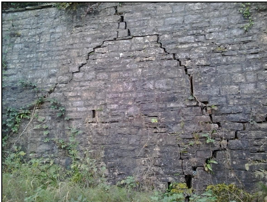
Plate 2.1. Cracking in retaining wall.
