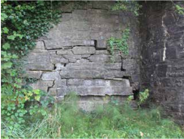
Cracks in retaining wall
