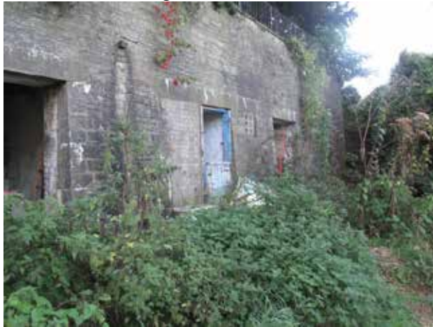
Sheds sunken into retaining wall
