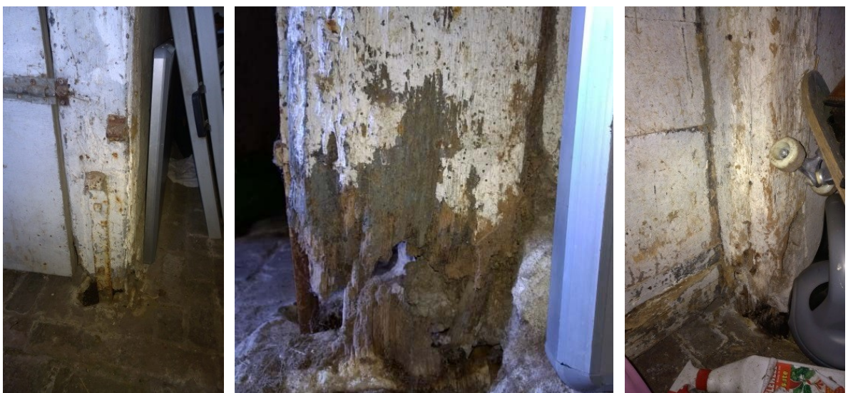
Figure 8 – Decay to base of existing posts
