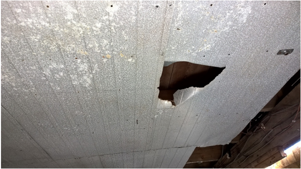
Photo 4: Hole in false ceiling with nesting material present at edge, possibly a pigeon nest.
