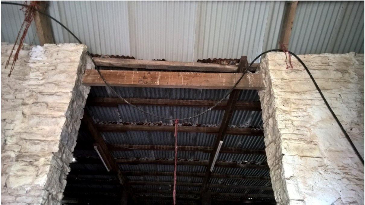
Photo 8: Pigeon excrement present on beam and on floor below. No nests were visible in this structure at the time of survey.
