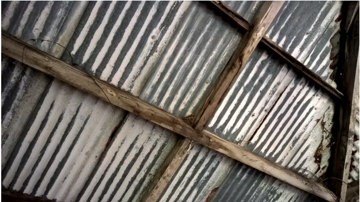
Photo 6: Old/currently disused nest at intersection of two beams in stable block.
