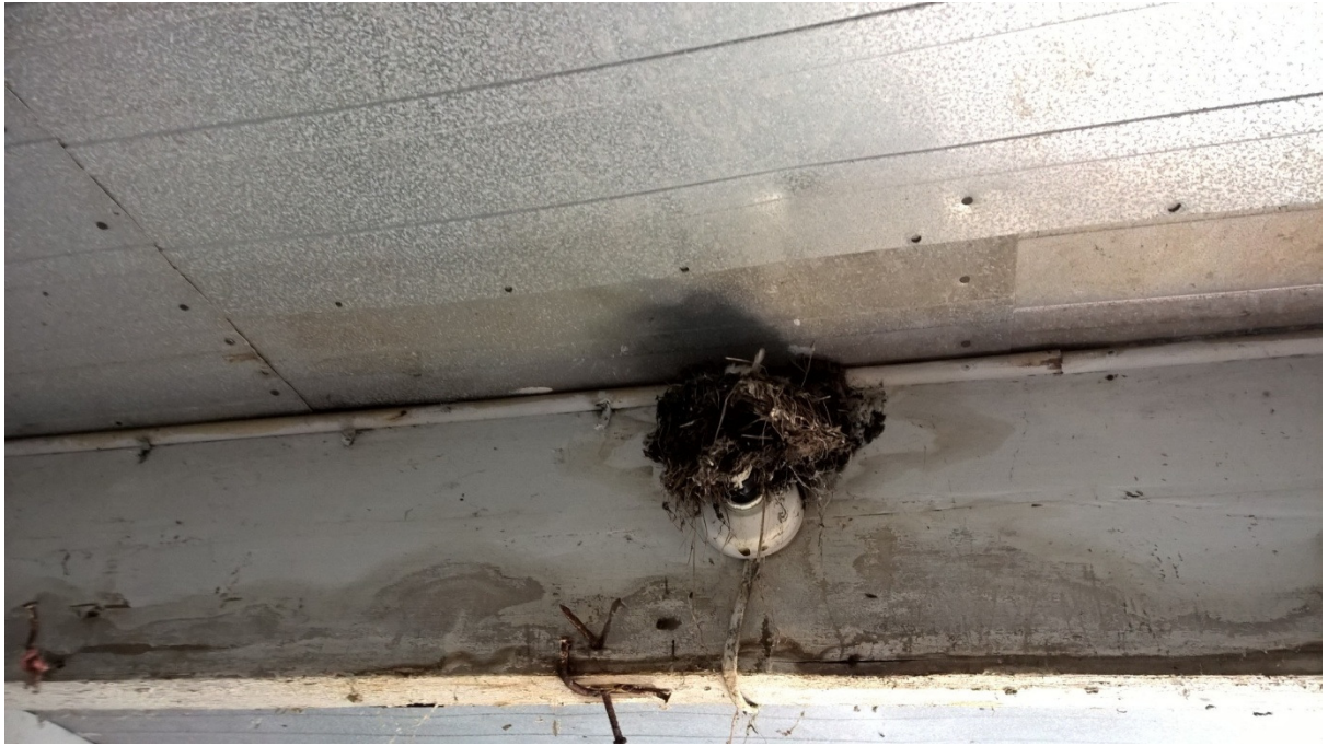
Photo 2: Currently disused/old swallow or house martin nest in lower storey of structure.
