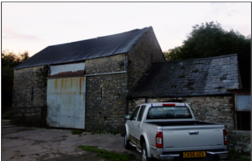
Stone Barn with Pipistrelle roost at the apex of the gable end.
