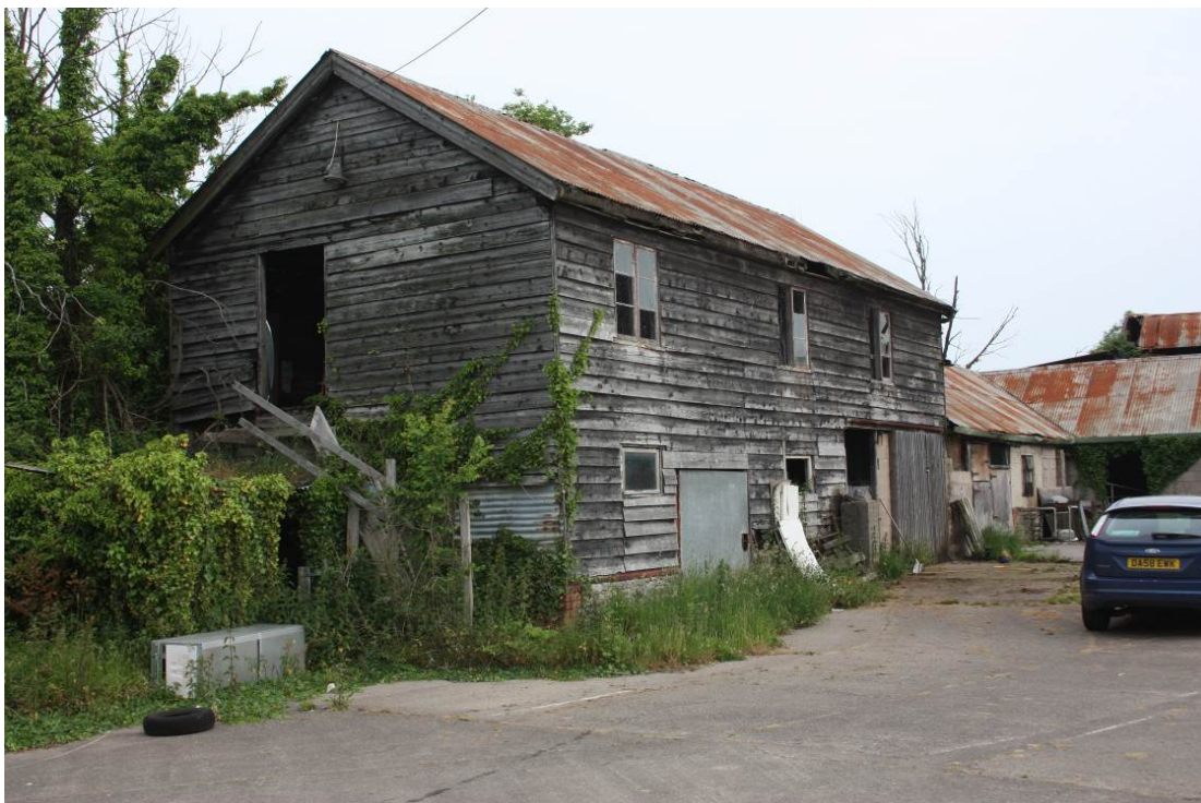
Image EDP 6: View of the barn at Greenyard Farm from the south east – here showing the existing (external) means of access to the first floor hay loft
