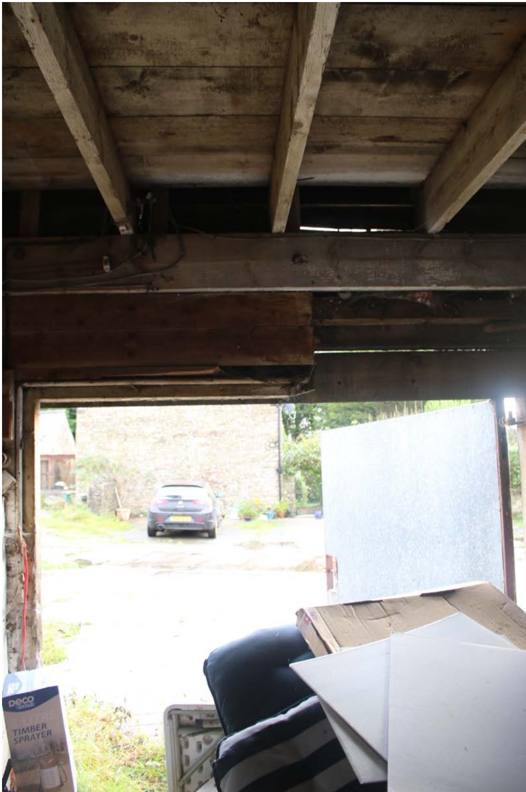
Image EDP 11: View out through the main door of the stable block; here illustrating its low height in comparison with the typical horse
