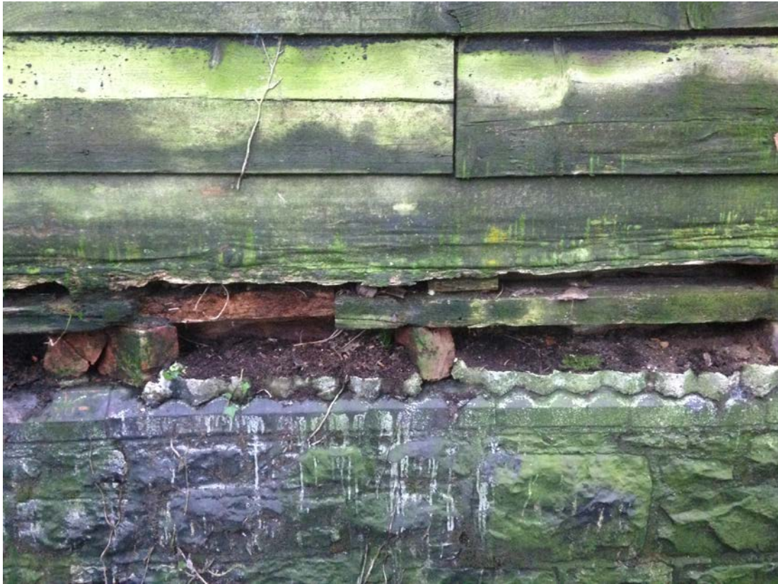
Image EDP 12: Close-up showing the relationship between the timber sill beam and the stone and red brick dwarf wall at the rear of the barn; clearly highlighting the use of basic materials
