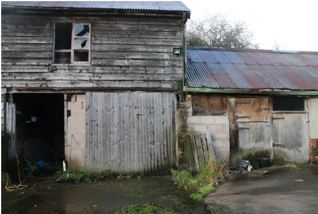
Image EDP 5: Close-up of the north end of the barn at Greenyard Farm; here illustrating that the north wall of the late 19 th century building is supported on concrete blocks
