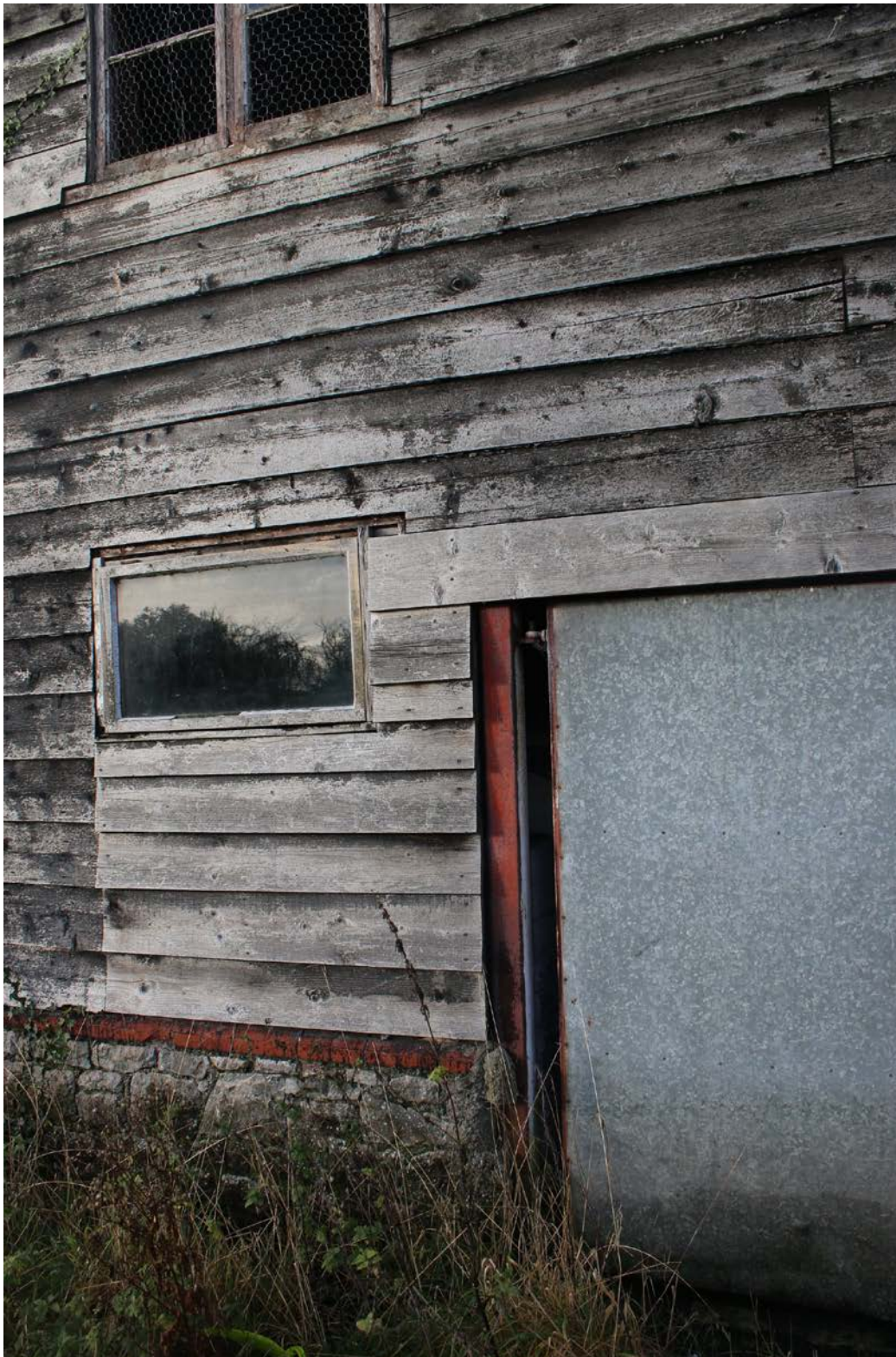
Image EDP 9: Close-up of the south side of the main door opening; here illustrating the ragged edge defined with concrete, strongly suggesting that it has been widened in the 20 th century
