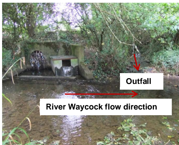
Figure 15.4 Outfall of unnamed watercourse into the River Waycock
