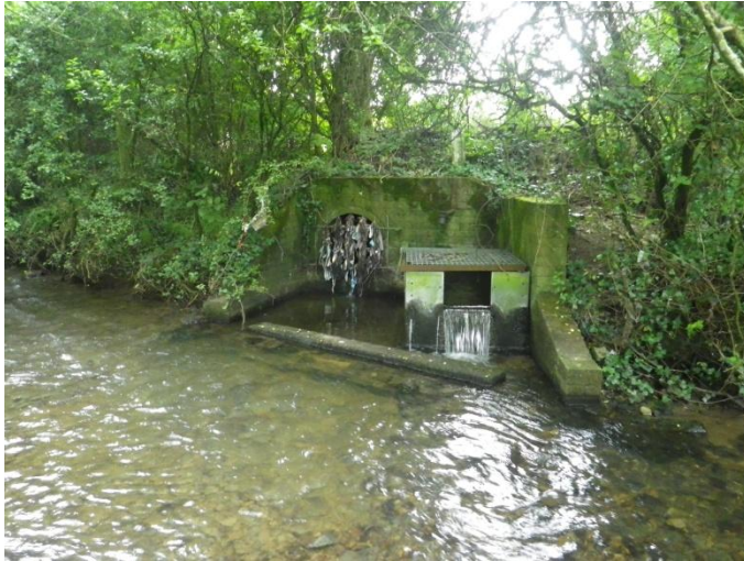
Photograph 7. Outflow from Waste Water Treatment Works upstream from bridge.
