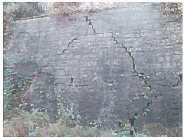
Cracks in retaining wall
