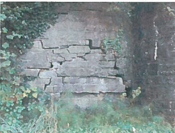
Cracks in retaining wall
