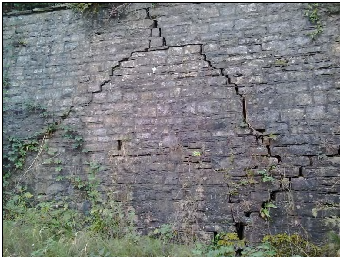
Plate 2.1. Cracking in retaining wall.
