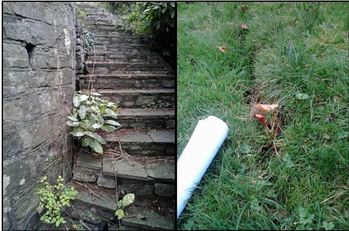
Plate 2.3. Evidence of Ground Movement during October 2015 visit.
