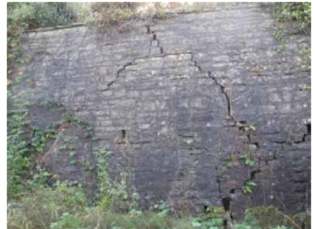
Cracks in retaining wall
