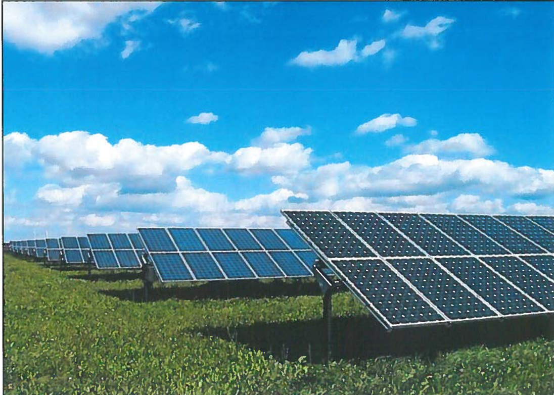
Figure 2: Photograph of Typical Panel Array (N.B. indicative of typical panels only)
