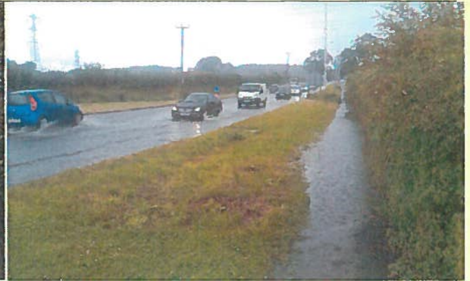
Footpath prone to flooding (2014)
