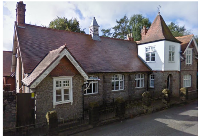
Example use of dark red/brown clay tiles in St. Nicholas and the use of decorative hanging tile on gables
