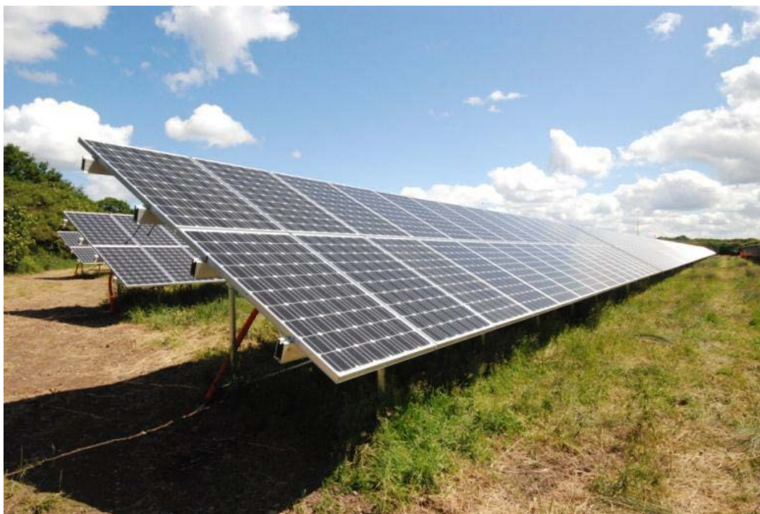
Image 2. Image of the likely design of the array and how the panels will be mounted
