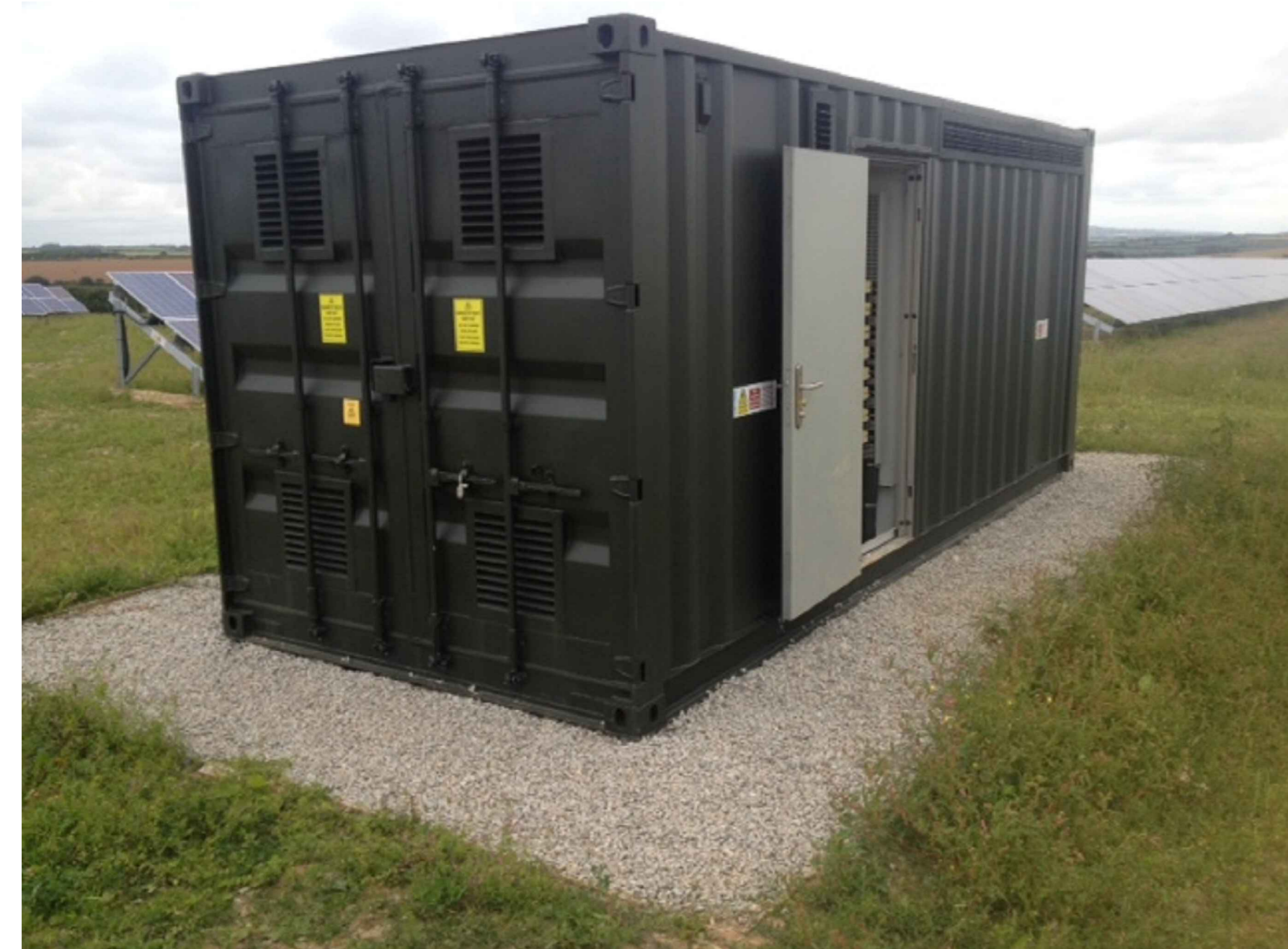
SWITCH ROOM TYPICAL EXTERNAL VIEW
