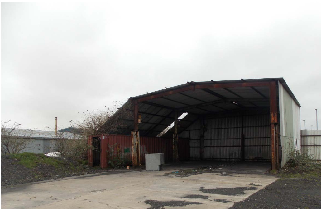
Image 6. Steel framed building to be demolished as part of the proposed works
