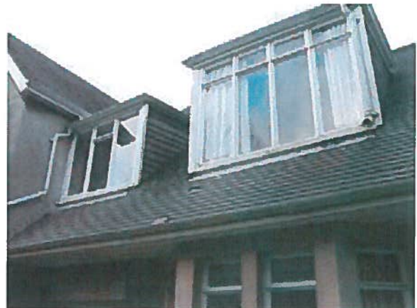
Dormer windows with slipped tiles visible
