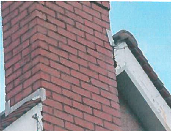
Gaps between fascia and chimney
