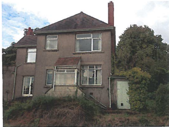
EXISTING FACADE - Strong dominant facade to the neighbouring dwelling, with tree buffer
