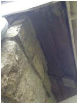
Figure 4: Gap beneath soffit box where single soprano pipistrelle entered
