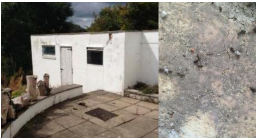
Figure 1: outbuilding (left) and old crumbling droppings characteristic of a pipistrelle species (right)
