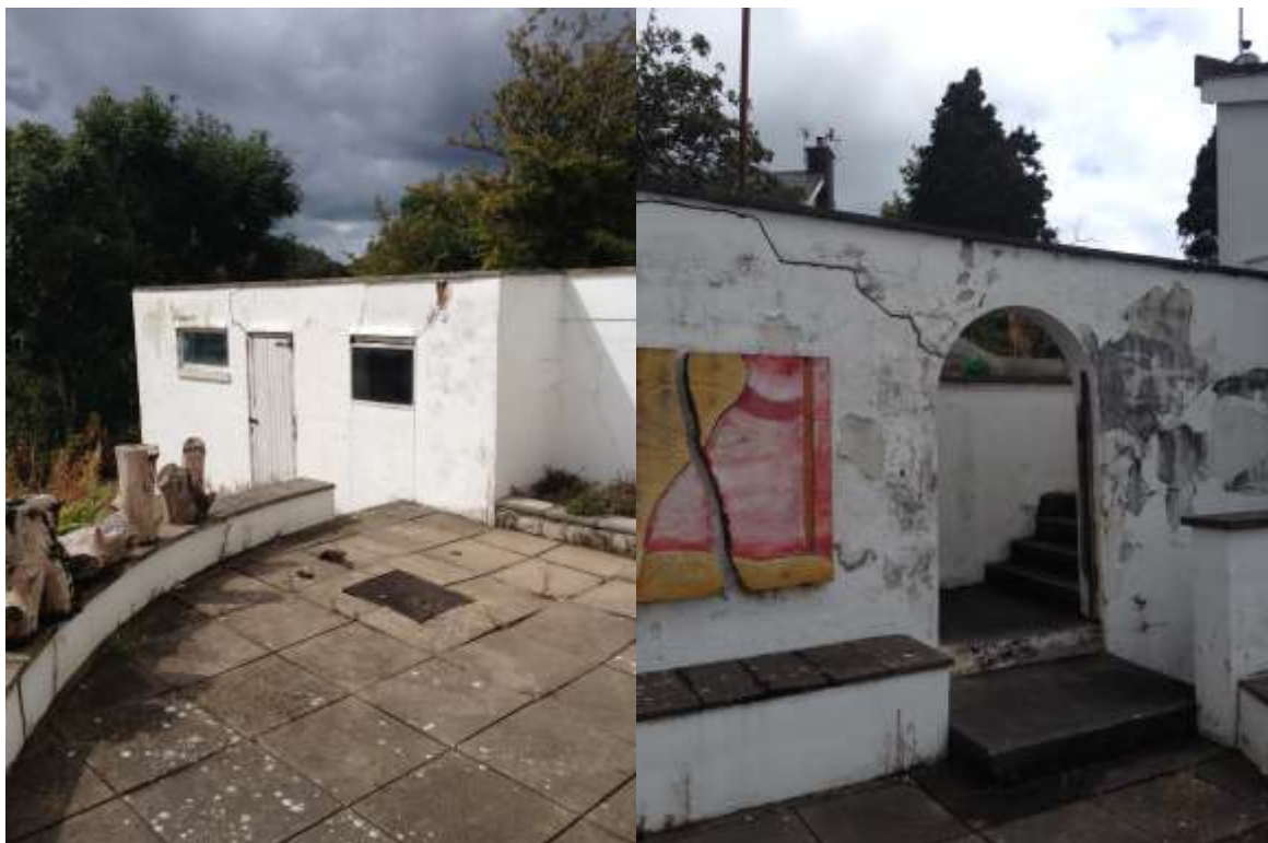
Fig. 14 &15 Storage shed and walled courtyard by pool. Note structural cracks.
