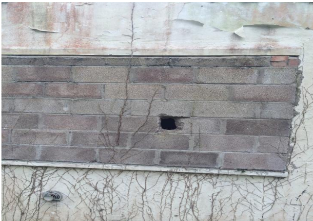
Plate 3: Hole in concrete blocks
