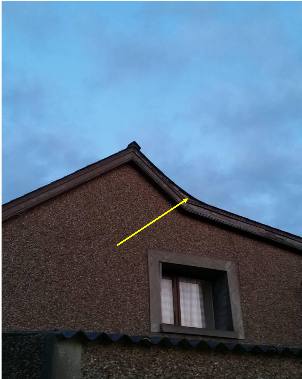
Plate1 - location of bat entry point on the eastern gable end of Welford Court Guesthouse
