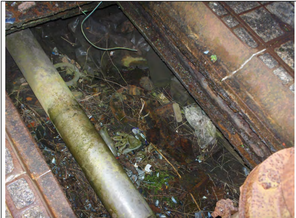
Plate 69: S/17633/19 Gasket in base of Duct
