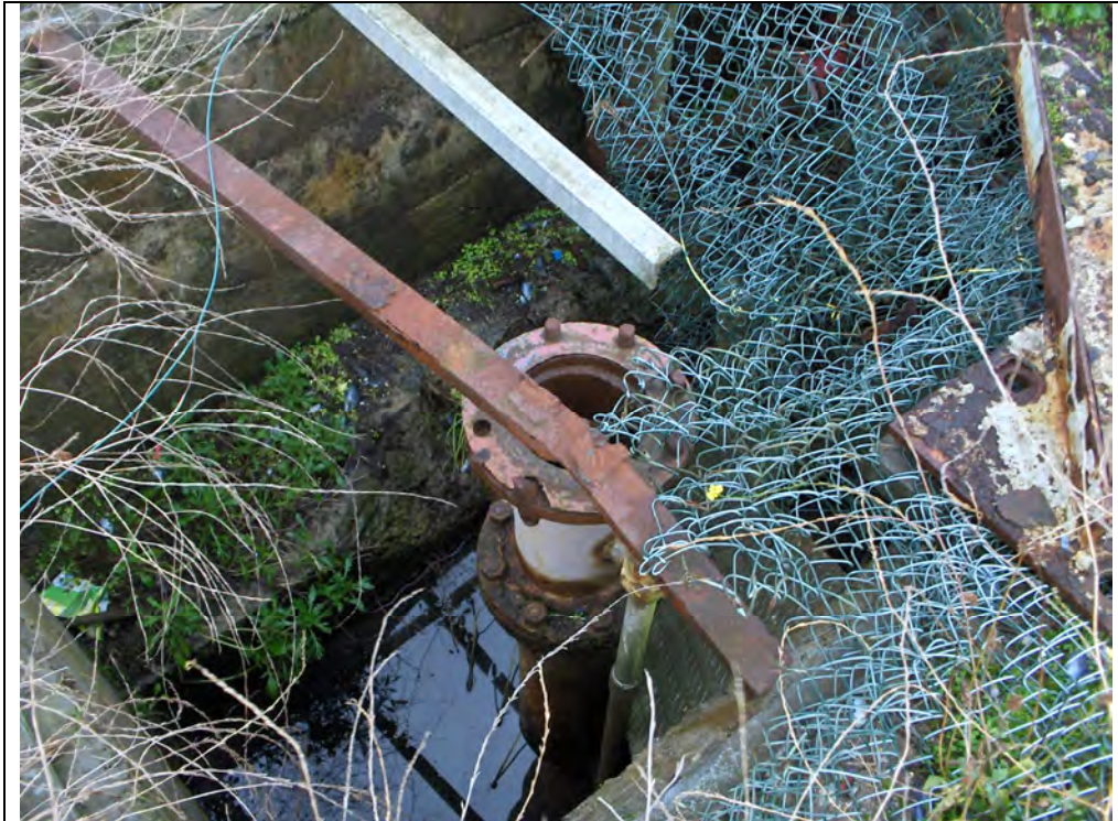
Plate 55: S/17633/05 Gasket to Pipe Flange
