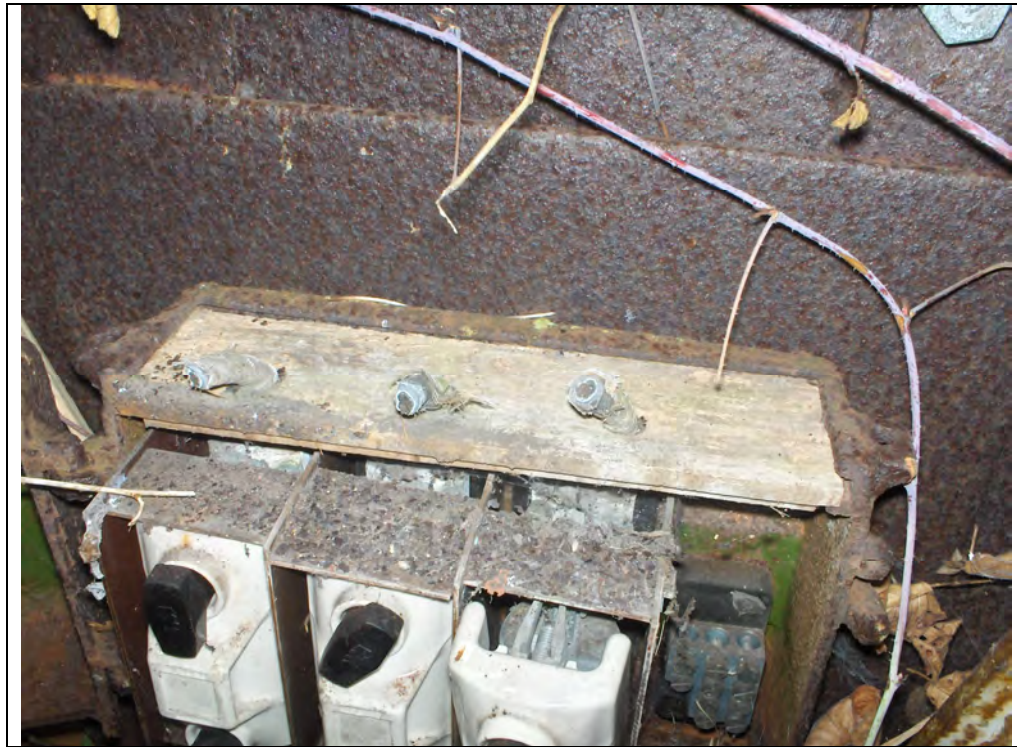
Plate 71: S/17633/21 Insulation Tape to Wire in Fuse Box
