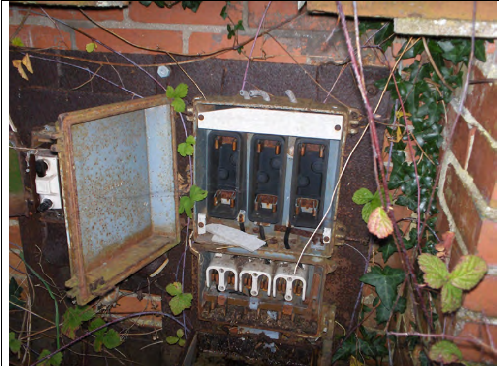
Plate 67: S/17633/17 Cement Flash Guards in Fuse Box
