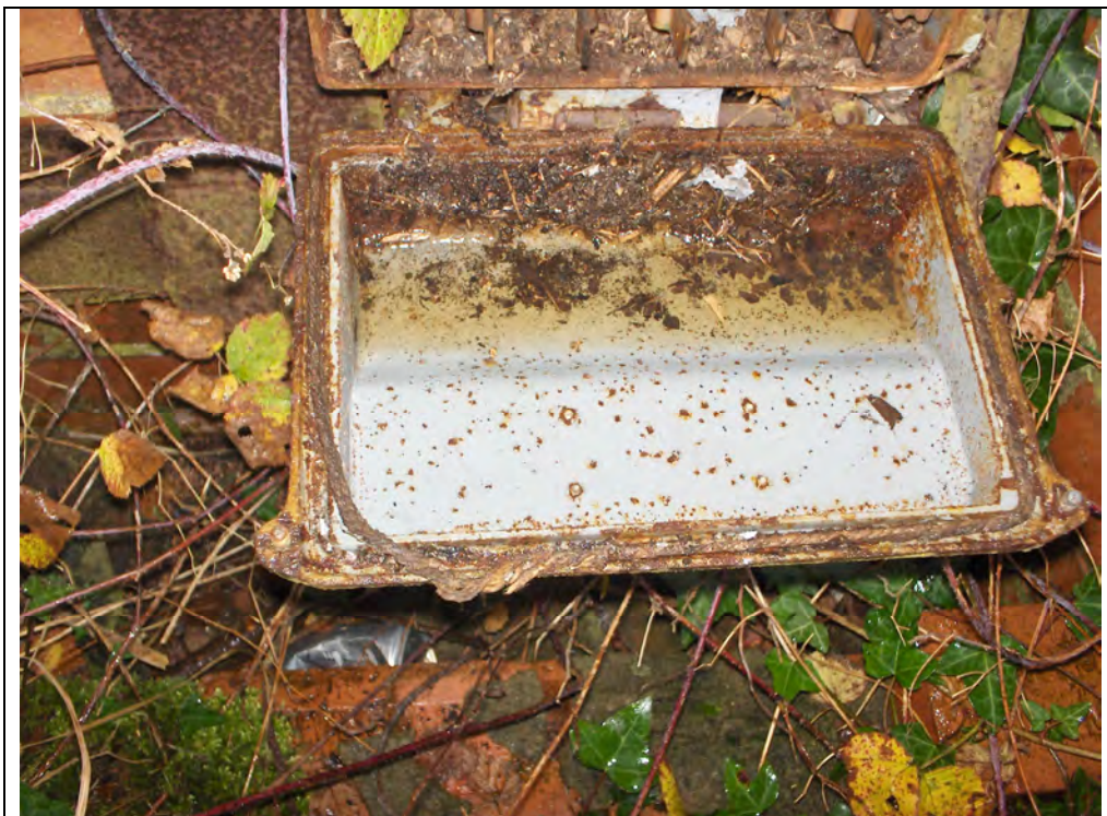
Plate 70: S/17633/20 Rope Gasket in Fuse Box
