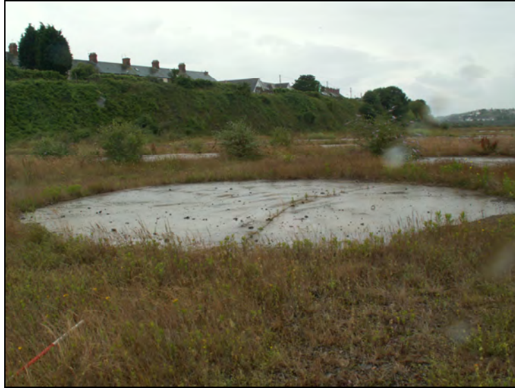
Plate G11: View to southwest of concrete tank base of Oil Storage Terminal
